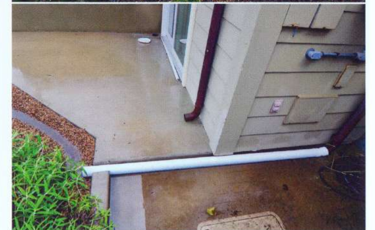
Above: A 4-inch curb cut allows hundreds of gallons of water to be filtered through the adjacent planter bypassing an area drain that once took water from a downspout directly to the storm drain at the Canfield's Indio Drive OFG.
