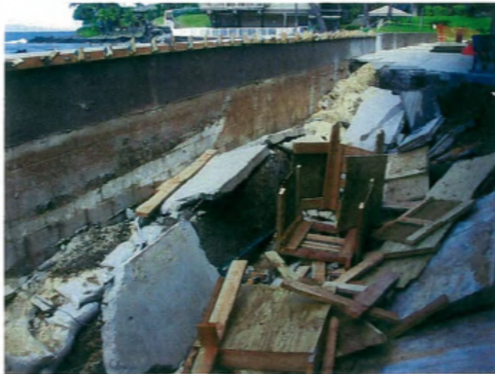
Unreinforced seawall fronting collapsed lanai area of Building F
